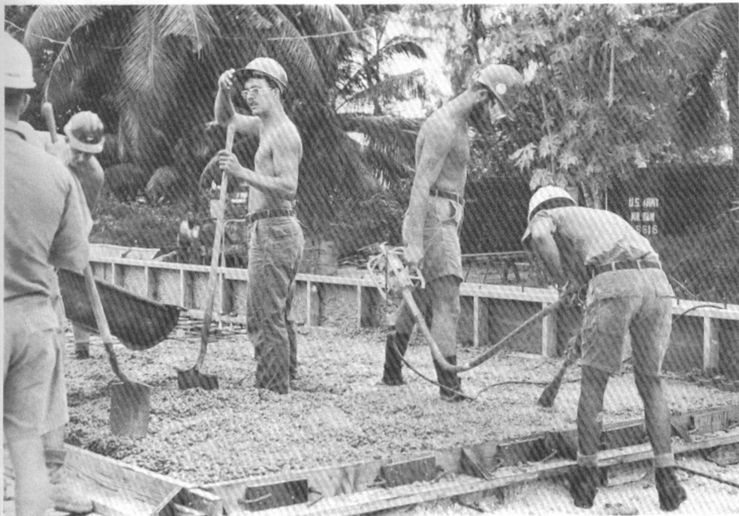
Seabees place concrete at the site of Diego Garcia's future swimming pool. The concrete is made of cement and crushed coral. (Photo by PH1 Robert Vaughn.)
