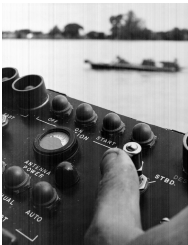
MSD Operation Console
